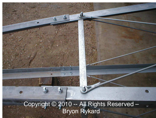
Figure 6a: Close up of the assembled topmost girt and "X" bracing (top view)
